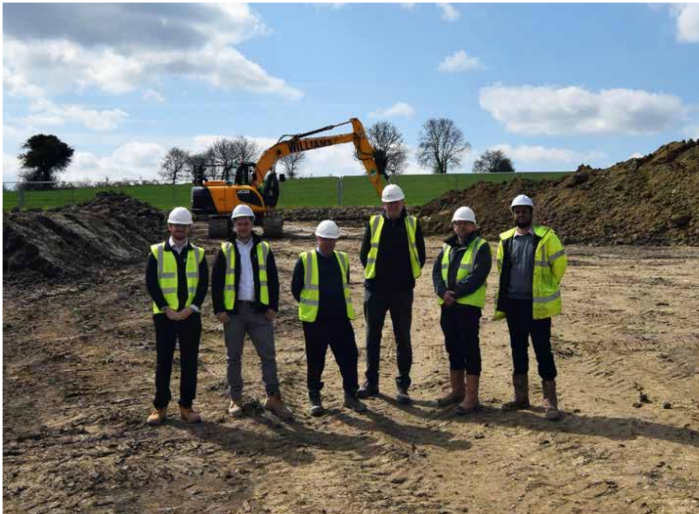
SWG Construction is building 14 homes at Callaughton's Ash, Much Wenlock, on behalf of Connexus
